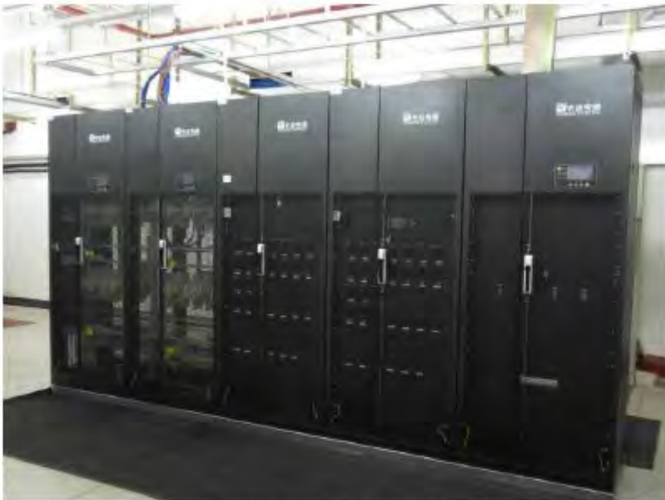
DC1+DC2+RC2+RC1+AC China Telecom
